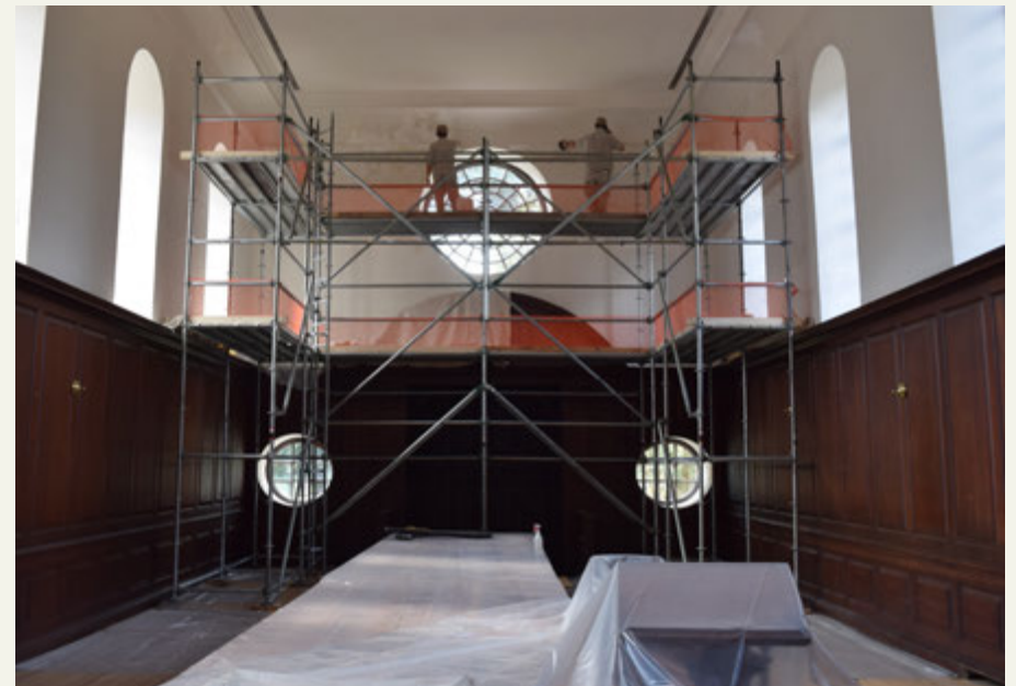
Scaffolding in the west end of the Great Hall allowed Colonial Williamsburg masons Chris Phaup and Isaac Hyde access to the upper wall and cornice on the south, west, and north walls of the room.
